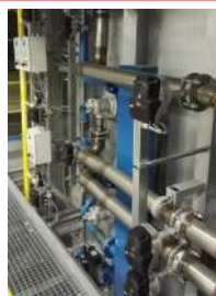
GASS, AIR PIPES
